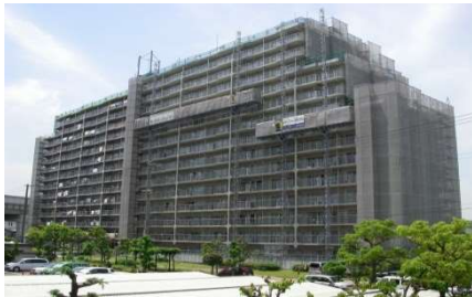
Repair work Repair works including repair, maintenance, etc. of buildings, bridges, and ultra-high-rise buildings
