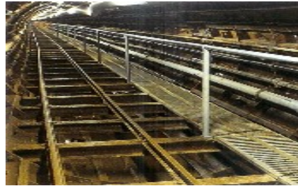
Underground work Shield tunneling construction such as subways, pipe lines, and utility tunnels
