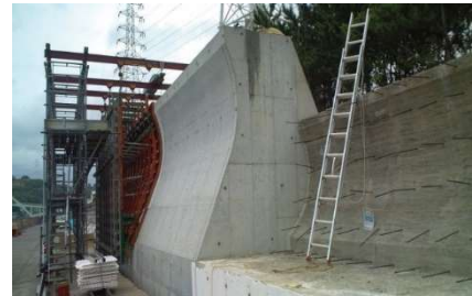
Ports (Breakwaters, etc.) Construction of breakwaters to prevent damage from high waves, high tide water and tsunamis
