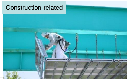
Hanging type scaffolding (Spider Panel) Walking panel hung with chains, mainly used in bridge repair work
