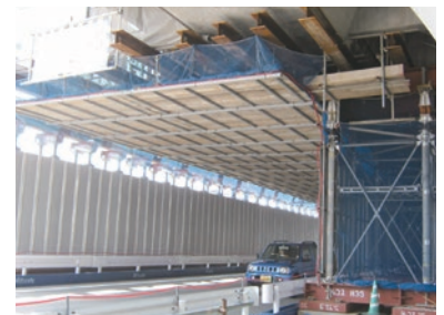
VMAX, hanging scaffolding system
